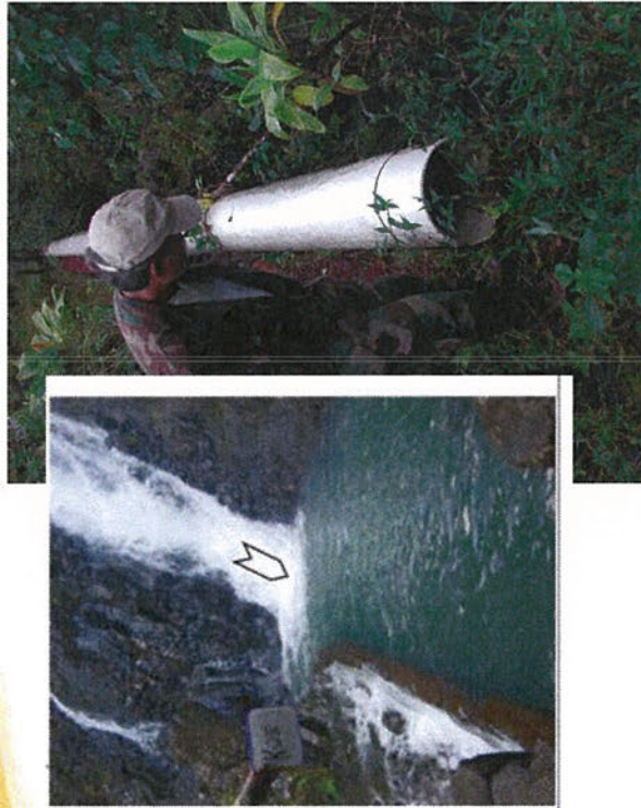
Main Kikokiko 6-in intake pipe - severed and no longer operational
